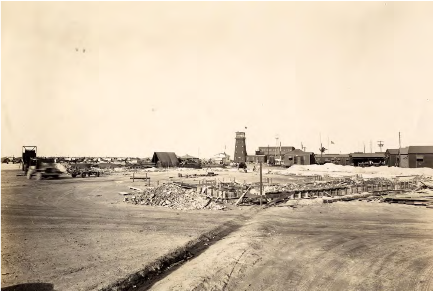
Foundation for hanger number 3 at NAAF Boca Chica taken on March 21, 1944. Photo credit: Monroe County Public Library.
