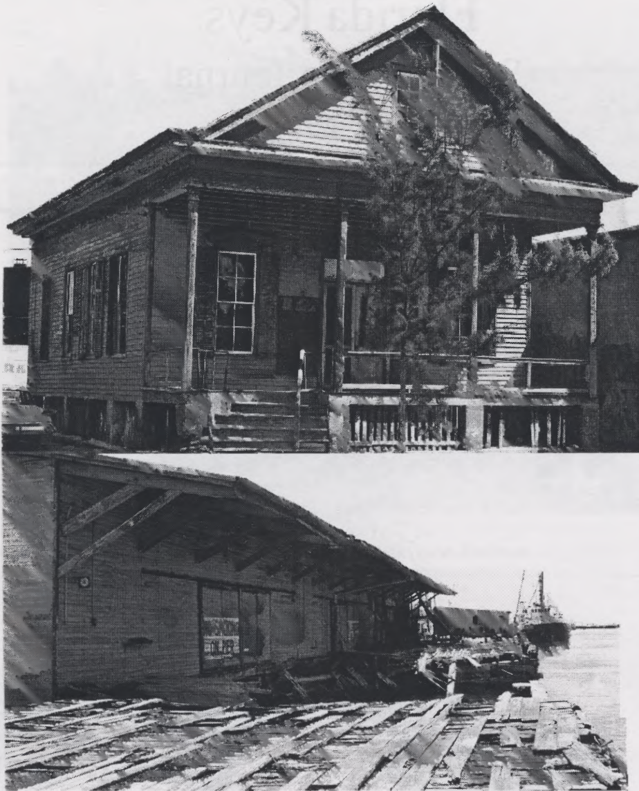
Hospitality House and Mallory Dock before restoration by Old Island Restoration Foundation. Photo credit: Monroe County Library.
