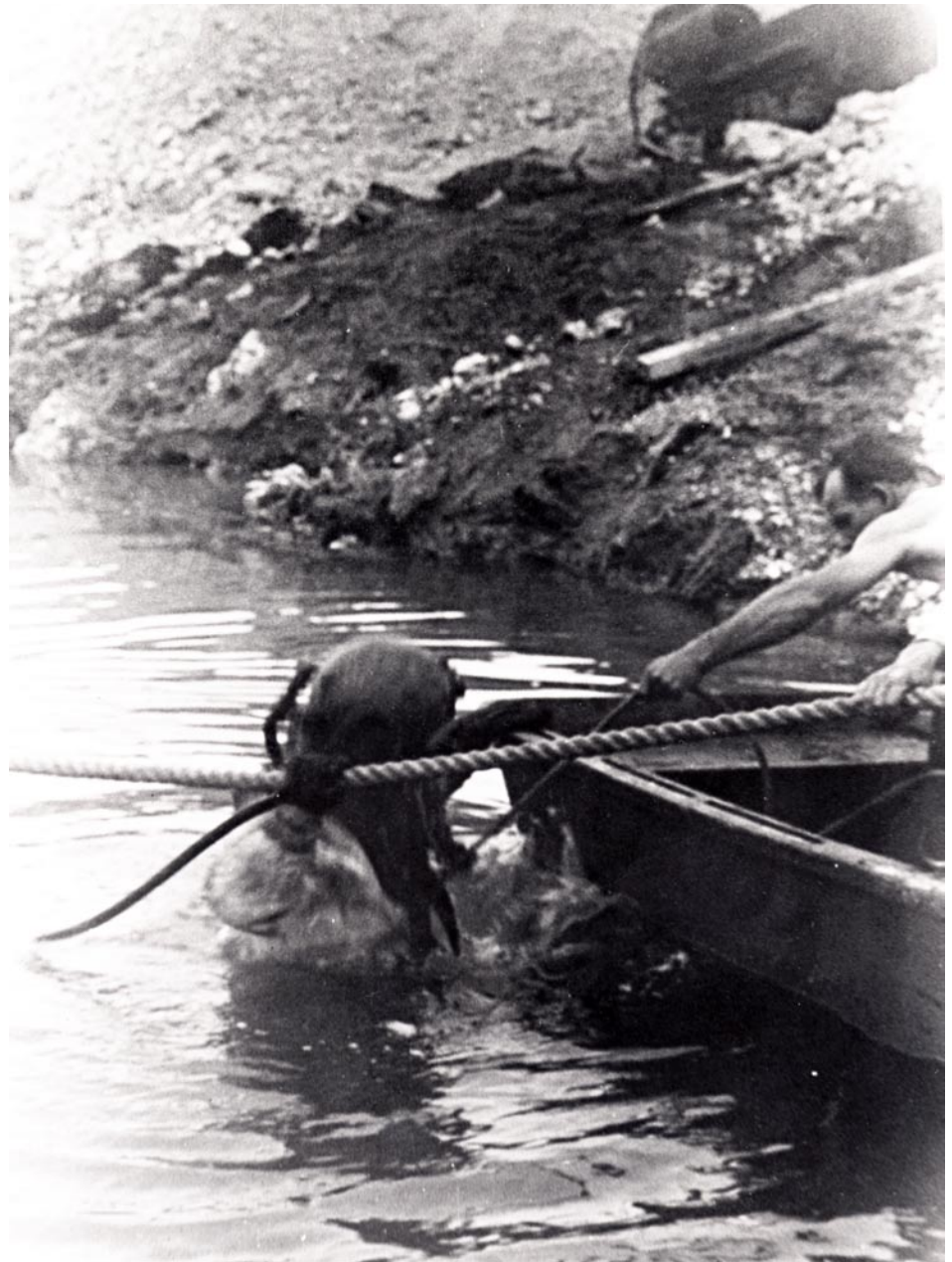
A haard hat diver working on the pipeline. Photo credit: Monroe County Library.
