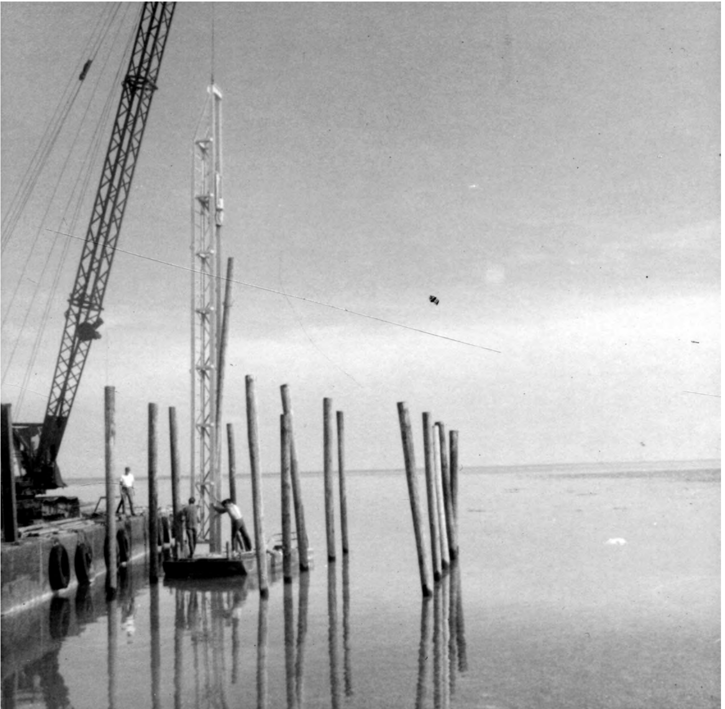
Captain Chet Alexander's Marine Salvage crew installing the pilings for the Koenig stilt house. Photo credit: Koenig Family.
